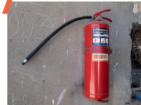
Fire extinguisher placement
