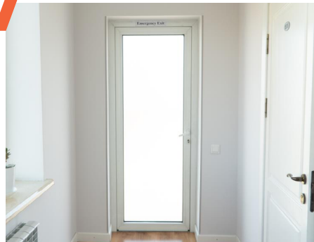
Access to the escape door must be free
